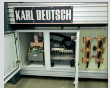
Field clamping switch (AC/DC for aerospace parts)
